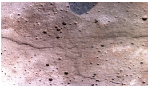
Figure 5. Crack Healing in the Specimen with Bacteria
