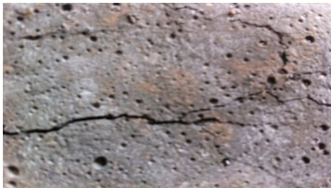
Figure 4. Crack Due To Manual External Loading
